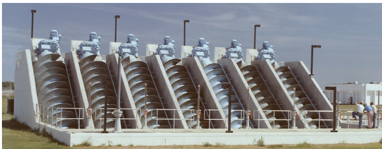
Seven Archimedes Screws pump wastewater in a treatment plant in Memphis, Tennessee. Each of these screws is 96 inches in diameter and can lift 19,900 gallons per minute. Source: Chris Rorres.
